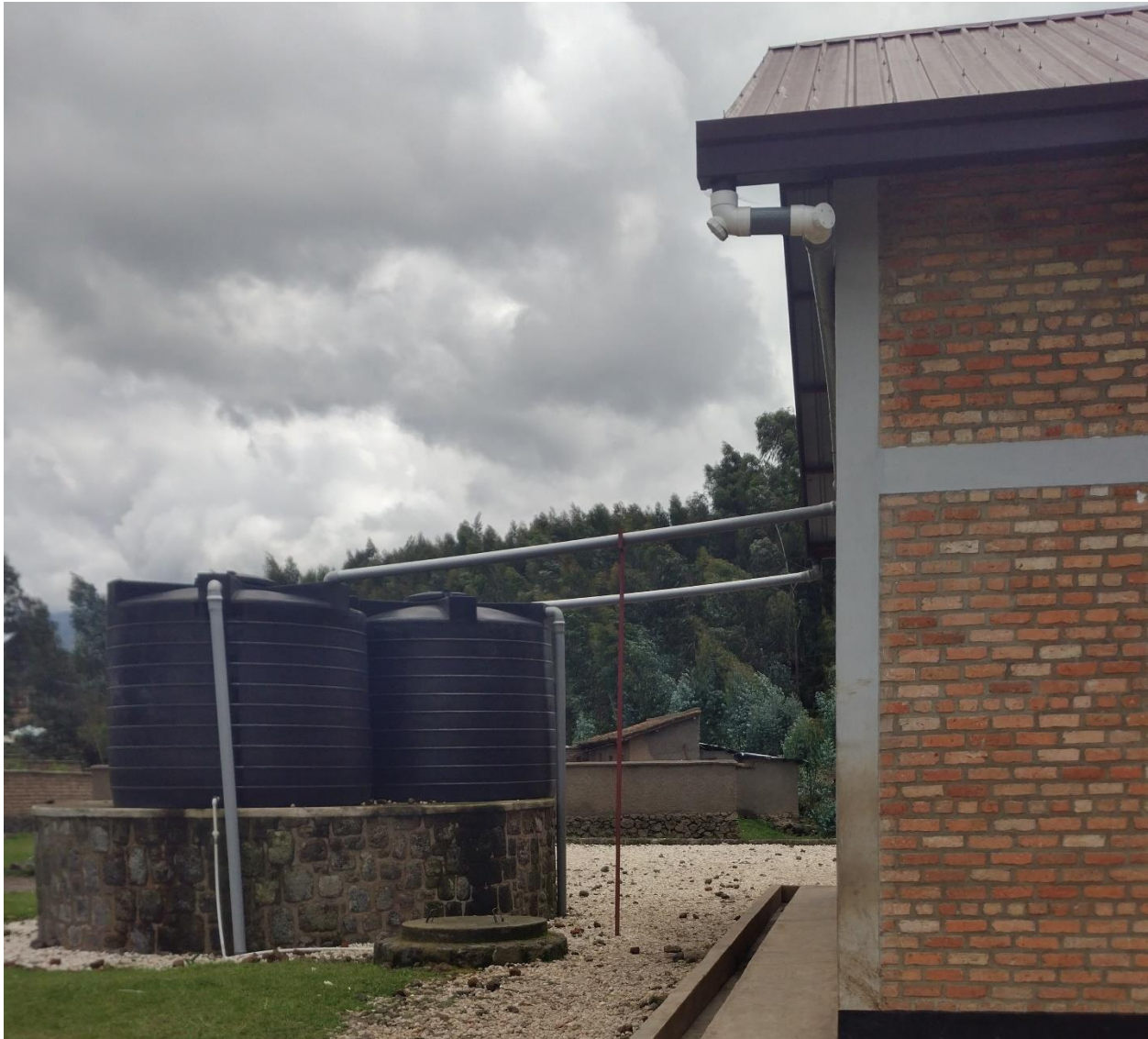
Photo 7 : RV3CBA Project also provided rain-water harvesting infrastructure
